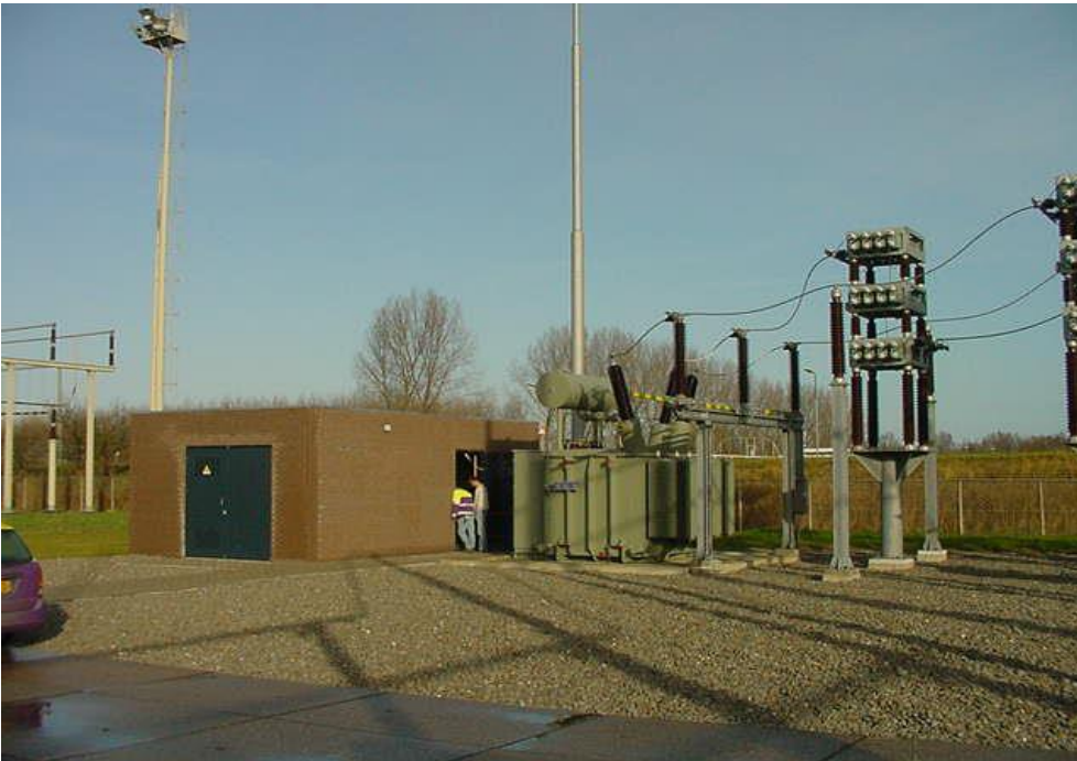
150 kV Coupling RAP (HV)
