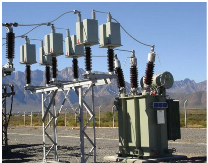
66 kV Coupling RAP (HV)
